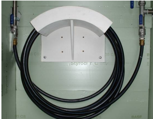
Figure II – Pipe coil in the plant
